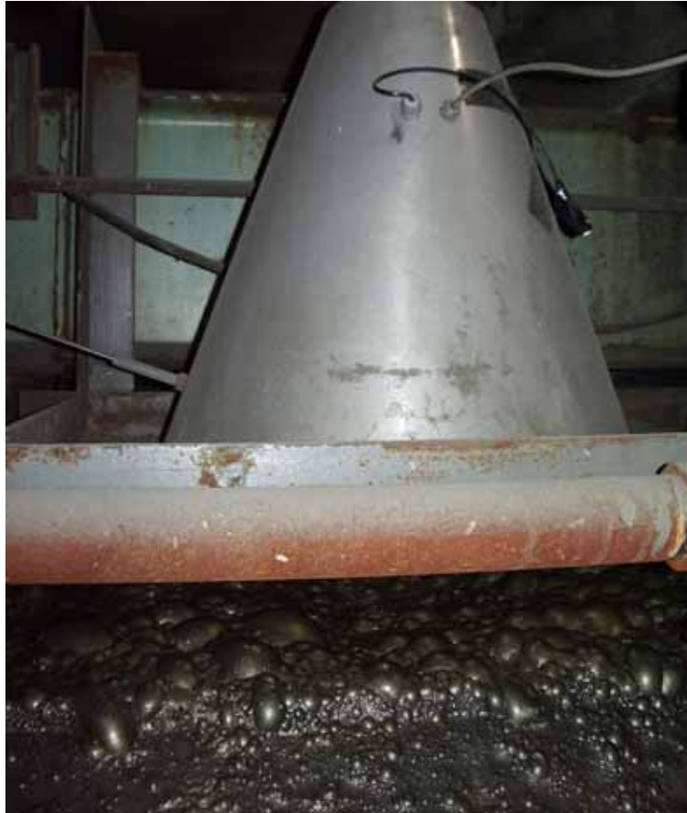
Figure 3.48: SmartFroth camera and hood system installed on cell 1, row 4 of the Kennecott copper circuit.
