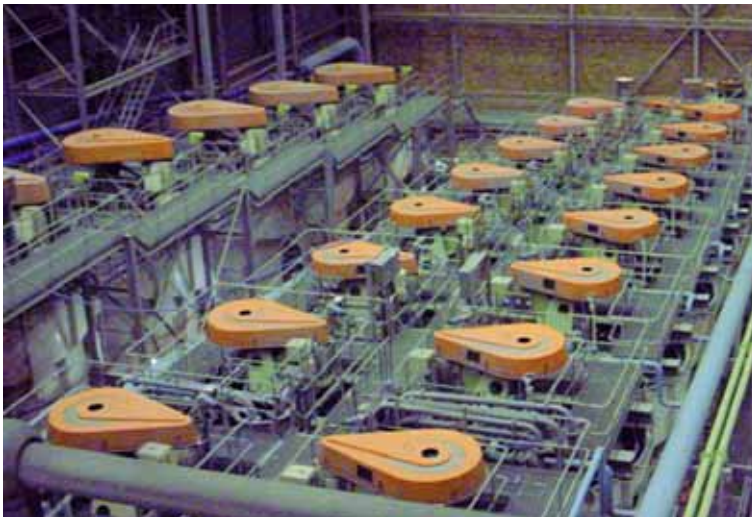
Figure 2.3: Three flotation banks on an industrial flotation plant.
