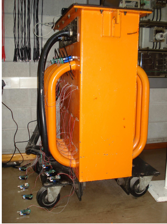
Figure 9.10: Isolation transformer with 15 sensor notes.
